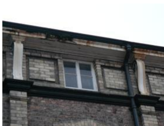
Photograph 23: Water Damage to Eaves 69 George Street
