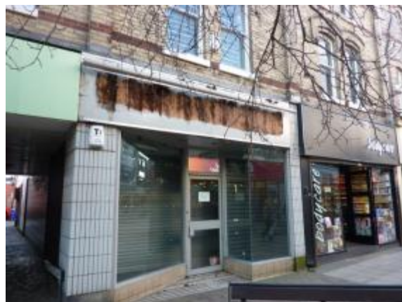
Photograph 14: Vacant Shop/Deteriorating Signage
